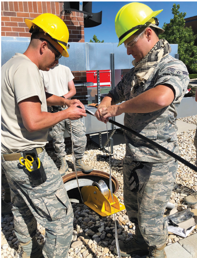
Tech. Sgt. Martin Montano (left) and Airman 1st Class Shane Miller pull fiber-optic cable to support communications and alarms for the munitions storage area at Gowen Field, Idaho.
